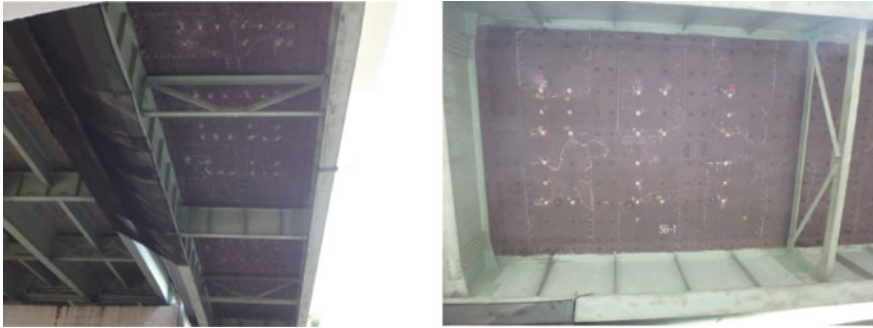
Fig. 7 Road bridge in service (left: general view; right: a panel in focus)
